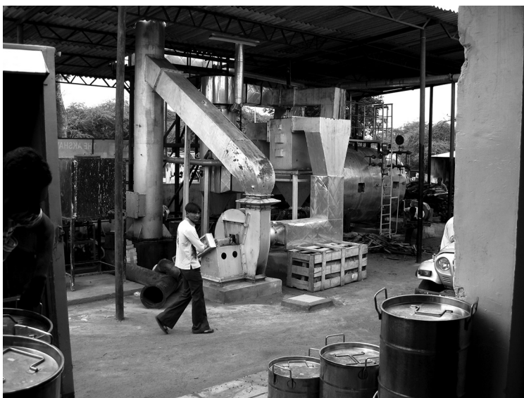
Figure A8.9 Boiler.
